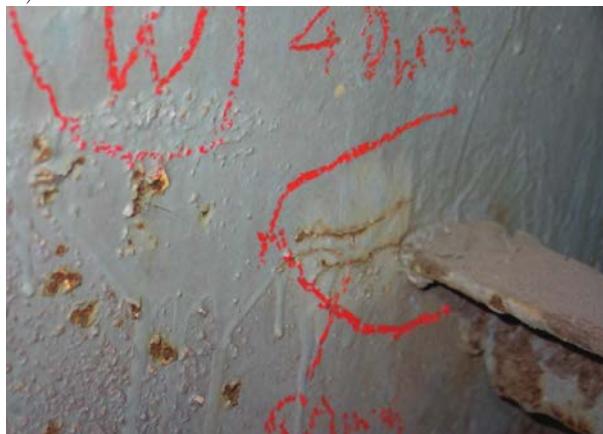
FIG. 5. Shell cracks above the long support: a) western side of the bridge – 80 mm and 45 mm long, b) eastern side of the bridge – 80 mm and 45 mm long.
